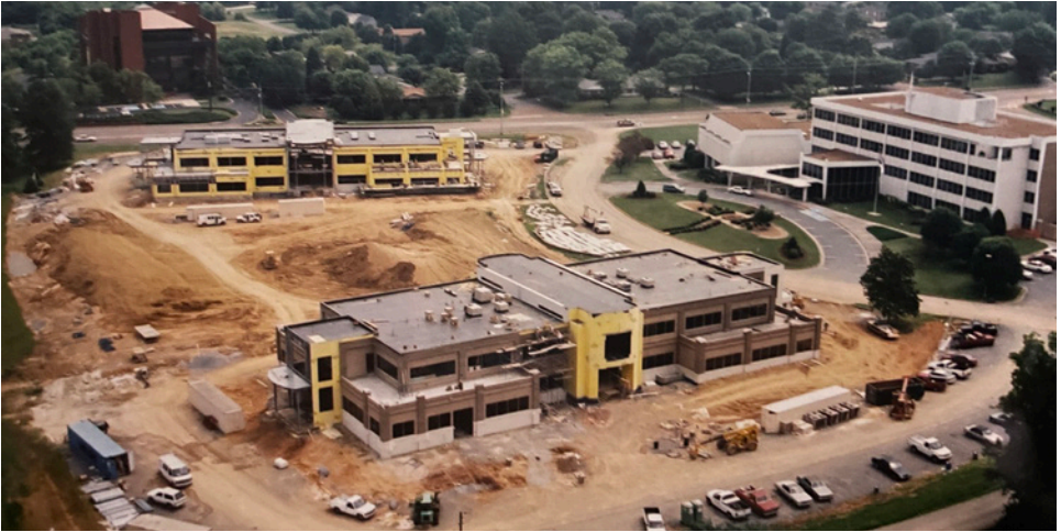
The Leadership and Communications Center (lower) and Discipleship and Education (upper) buildings under construction as the future World Evangelism Center awaits renovation.
